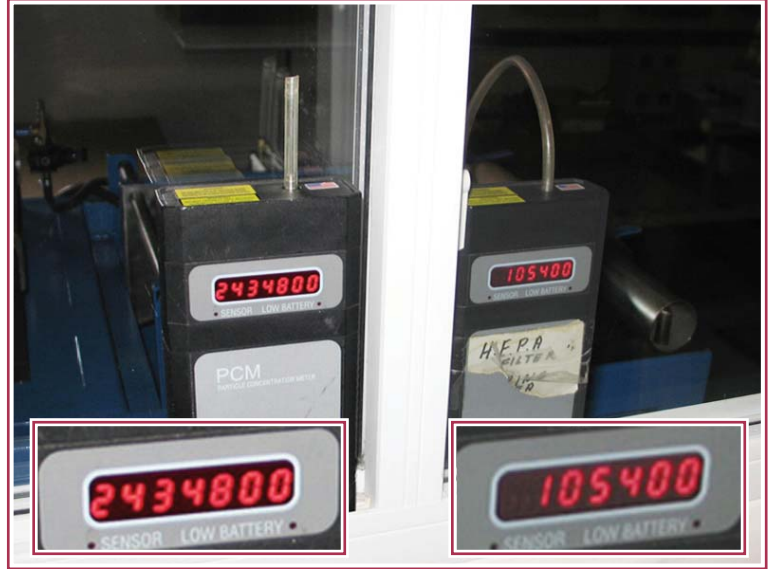
Above Left: 3 Amaircare ® 2500HVs installed above Cleanroom.
